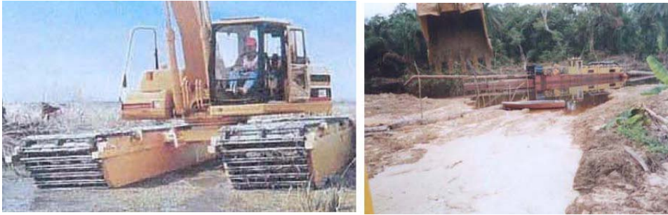
Figure 3b: Swamp buggy creating a path into the site for the dredger.
