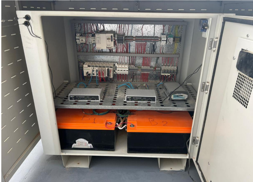
Figure 3: KSA-CORS Cabinet Components
