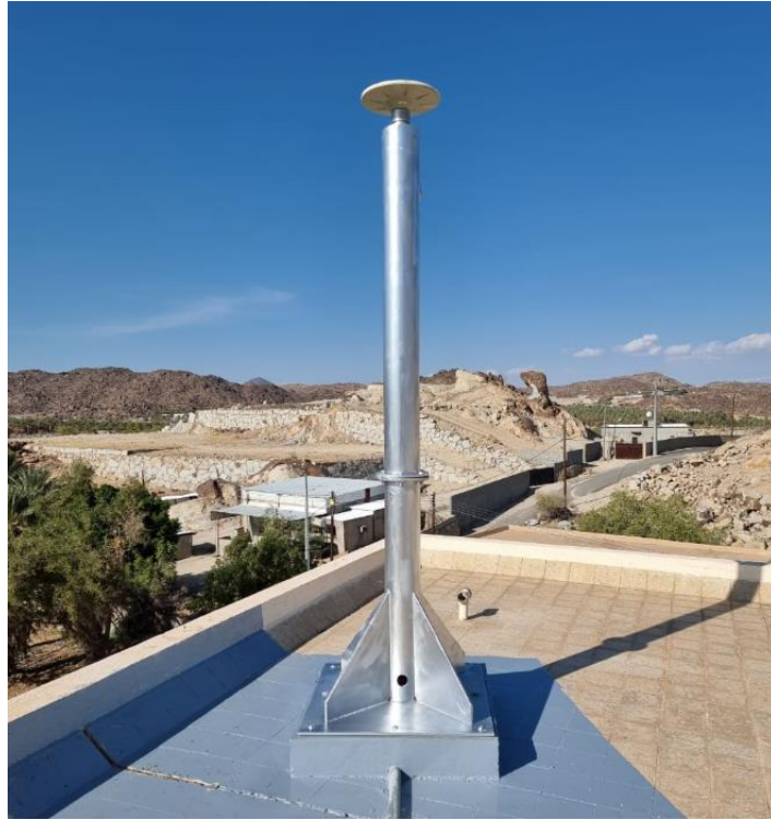
Figure 2: A typical KSA-CORS Roof Type station
