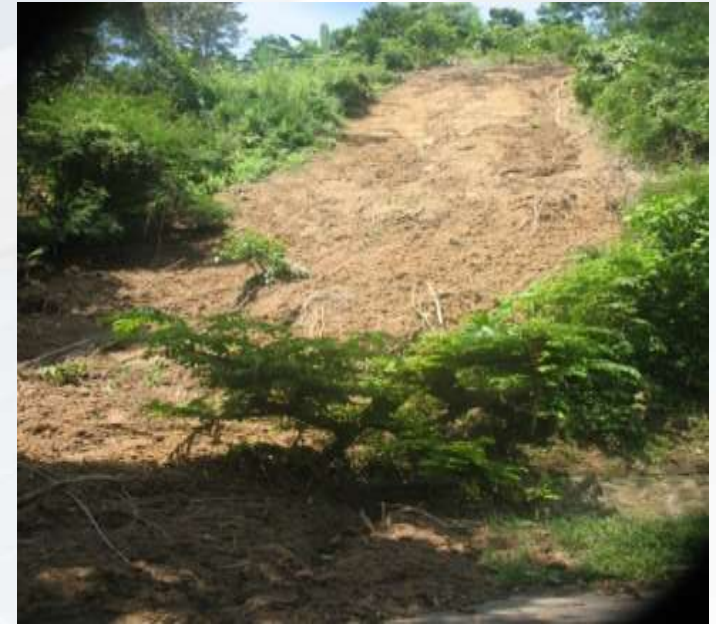
Massive landslides in the roadside Cipongkor-Saguling
