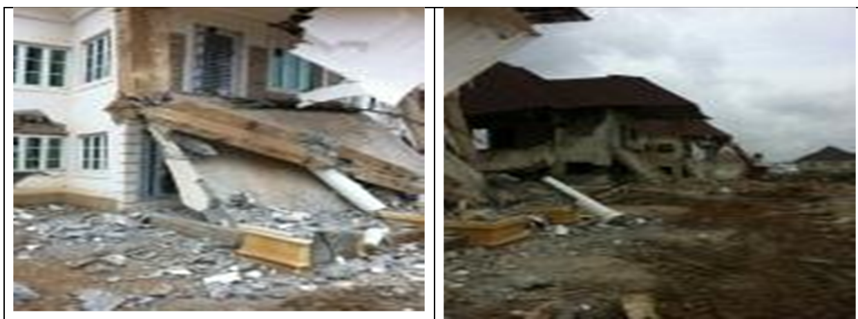
FIGURES 6 & 7: RESIDENTIAL APARTMENTS BUILT ON SCHOOL PLOT AND REMOVED BY DEVELOPMENT CONTROL DEPARTMENT
