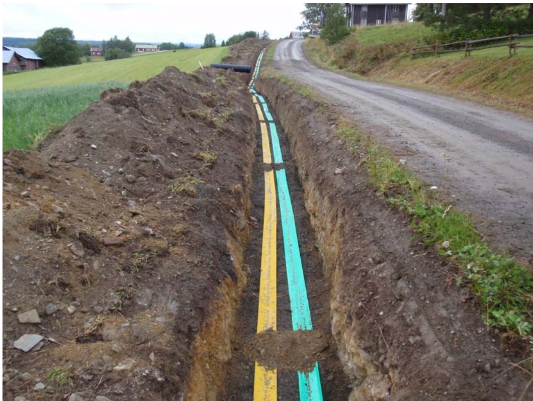
Cable ditch, electricity and broadband
