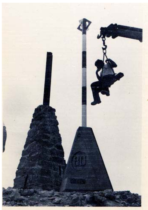
Fig. 22: A border pillar in the Egypt-Israel border after the 1982 peace treaty. On the left, the old border pillar from 1906 agreement
