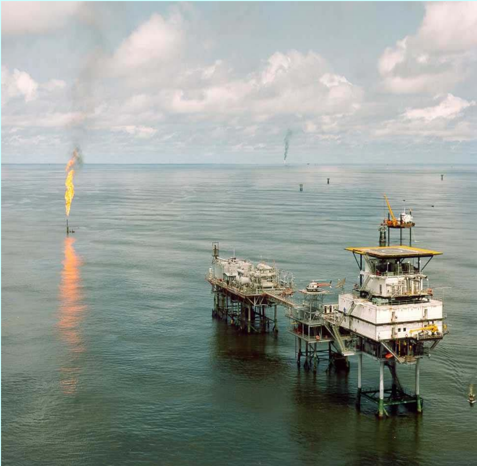
Figure 1: An Offshore Production Platform
